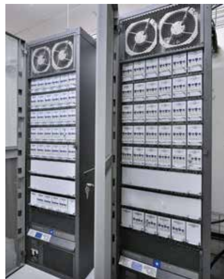
Armoires de gradateurs Philips Strand Lighting EC21 Dimming System
